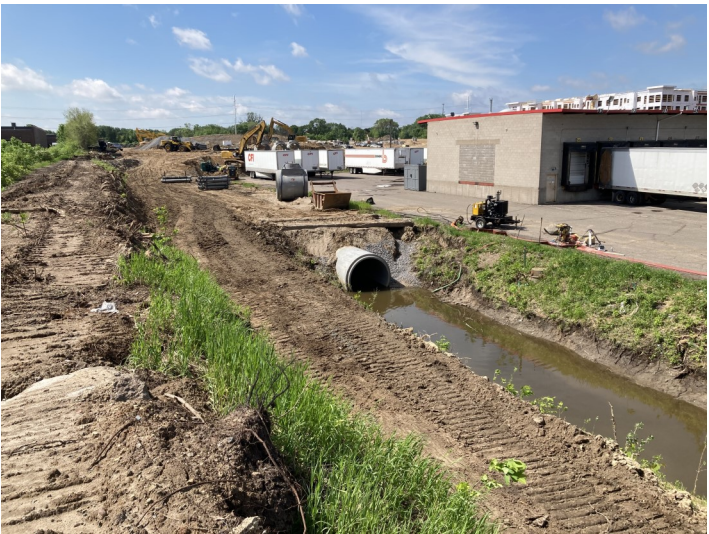
Downstream conditions following a rain event south of Terrace Dr
