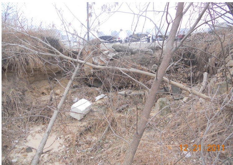
2011 photo identifying bank failure due to overland flow from an adjacent property
