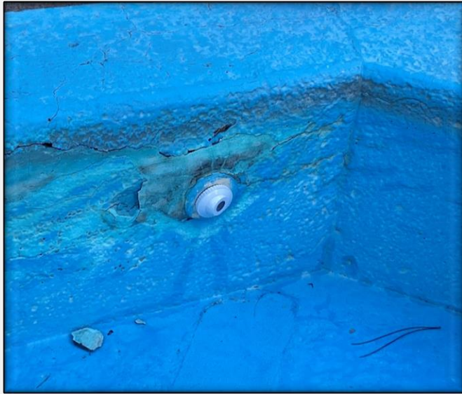
Cracked Piping In Recirculation System
