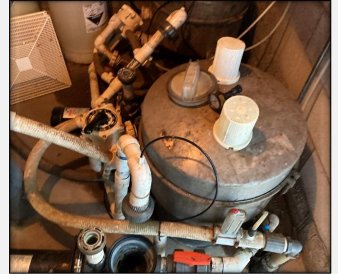
Outdated Filtration System
