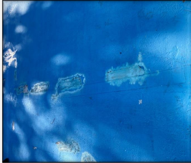
Cracking on Pool Floor
