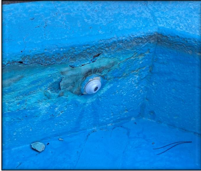
Cracked Piping In Recirculation System
