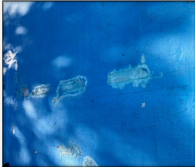
Cracking on Pool Floor
