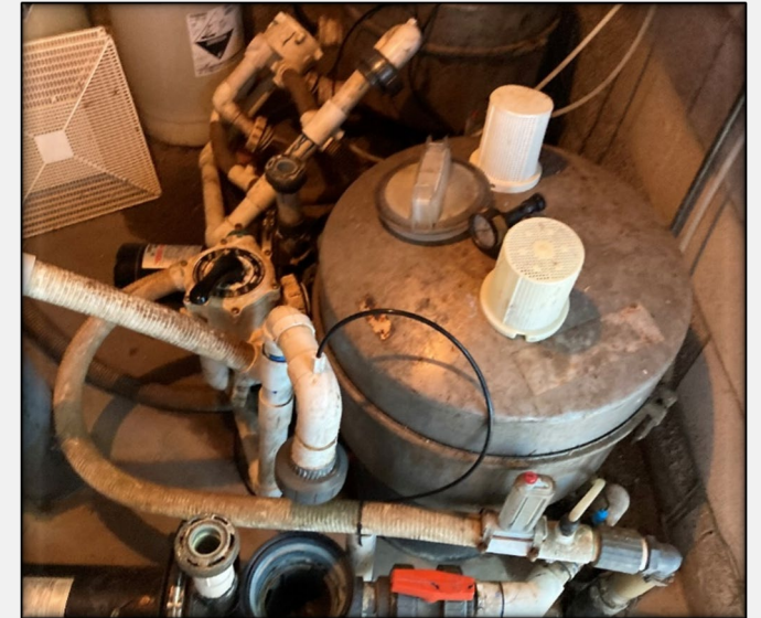
Outdated Filtration System
