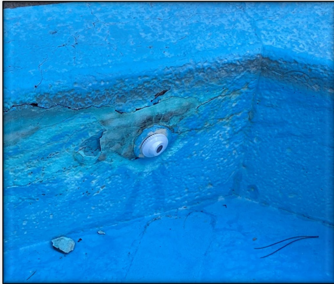
Cracked Piping In Recirculation System
