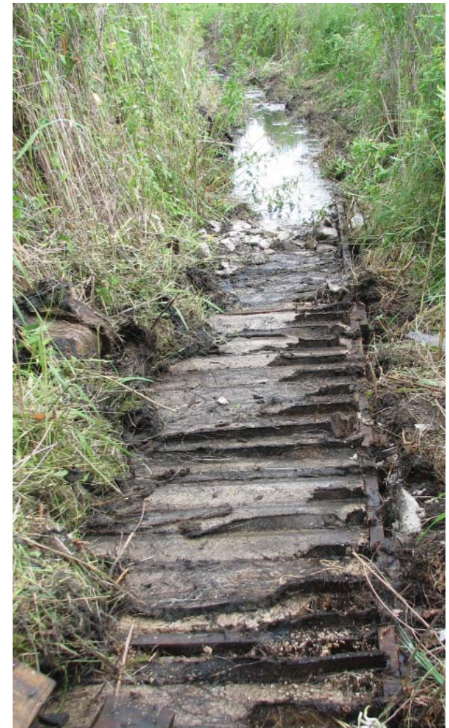
Components of a parks and recreation system are in need of constant attention, as wear diminishes the quality of the experience and can pose hazards for users. Every component of a system needs to be replaced someday.
