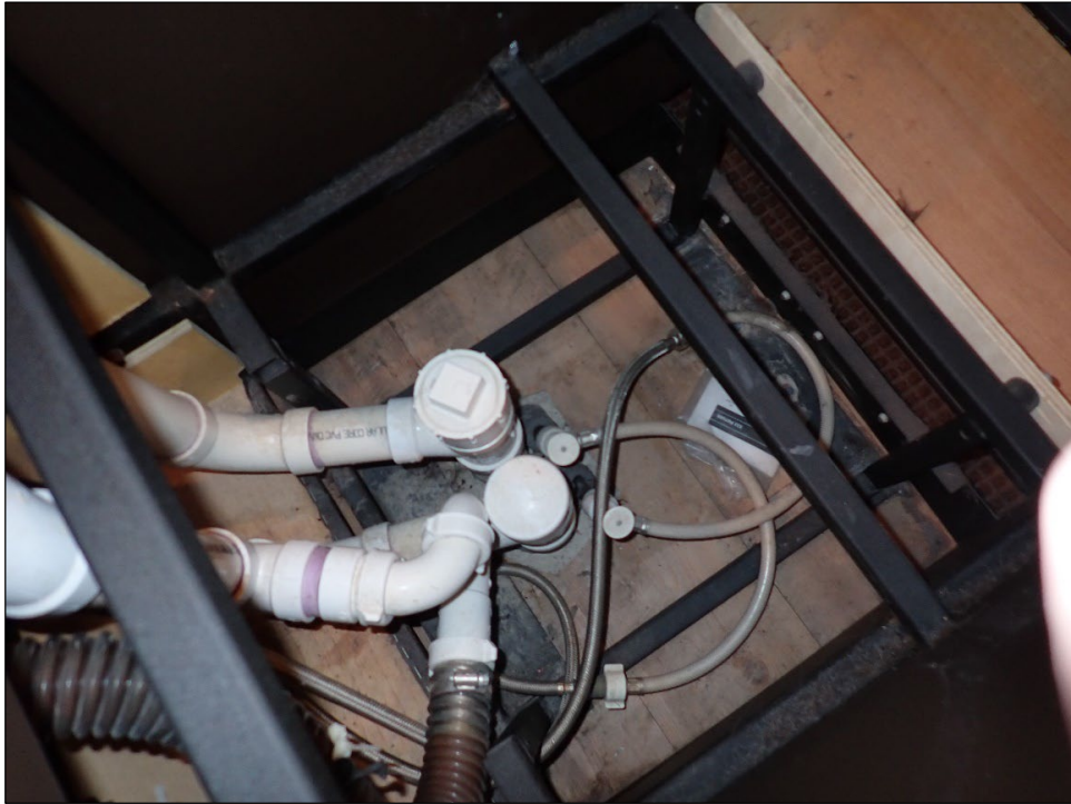
Plumbing Under Shampooing Chair (part of Item K)
