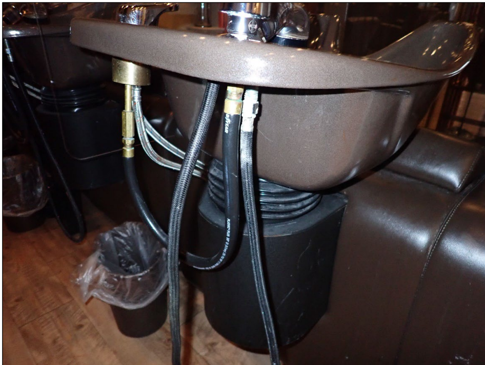
Integrated Sink on Shampooing Chair Note : Plumbing to Faucet (part of Item K)
