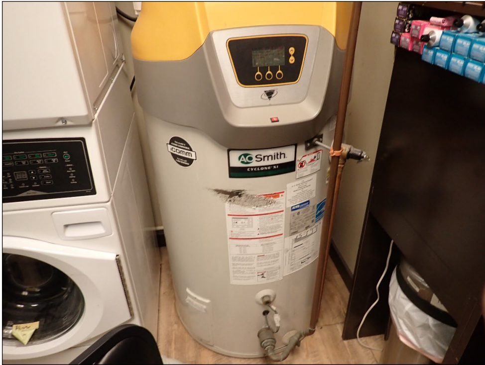
Item O - Water Heater
