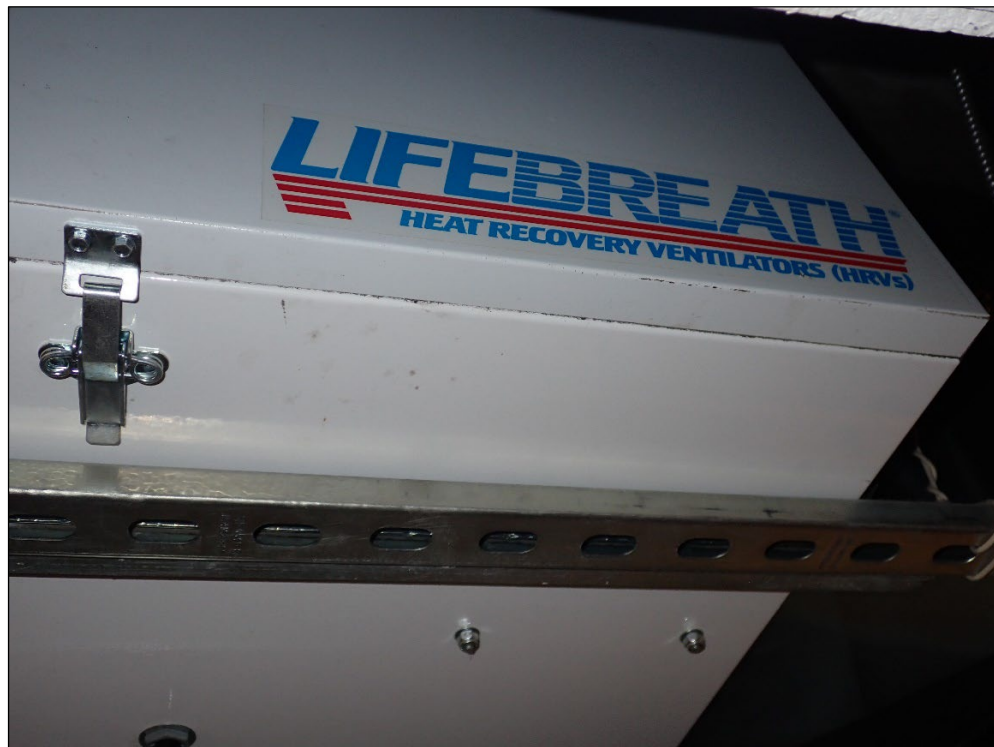
Item N - Heat Recovery Ventilator
