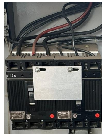
Main Service Disconnect
