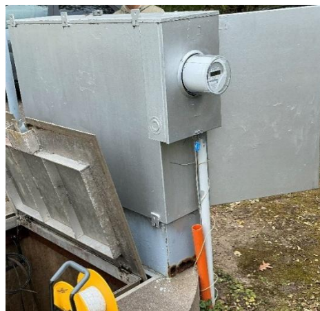
Control Panel/Utility Meter
