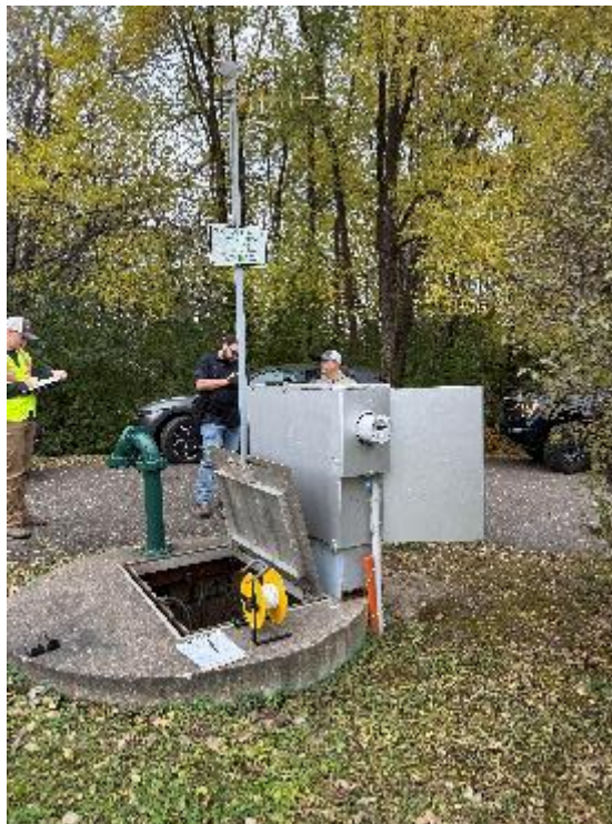
Figure 2.9: Brenner Sanitary Lift Station Wet Well Lid and Control Panel
