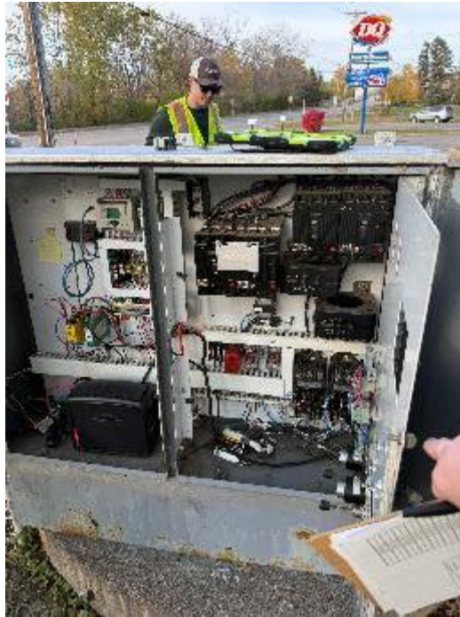
Figure 2.12: Brenner Sanitary Lift Station Control Panel
