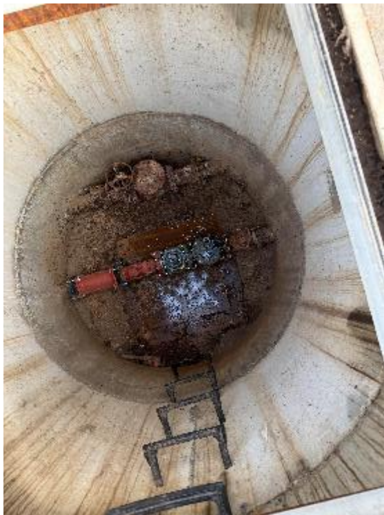
Figure 2.11: Brenner Sanitary Lift Station Valve Vault
