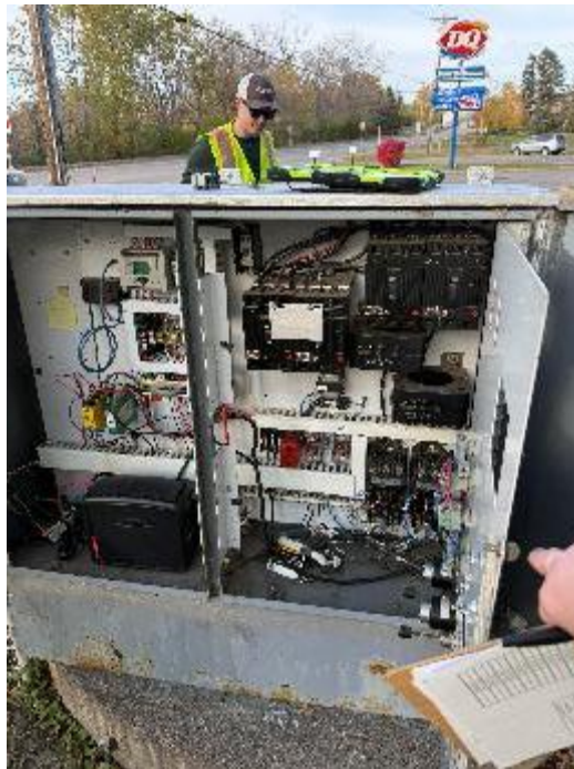
Figure 2.12: Brenner Sanitary Lift Station Control Panel
