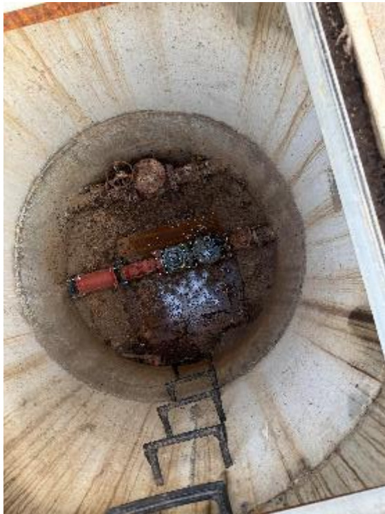
Figure 2.11: Brenner Sanitary Lift Station Valve Vault
