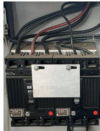
Main Service Disconnect
