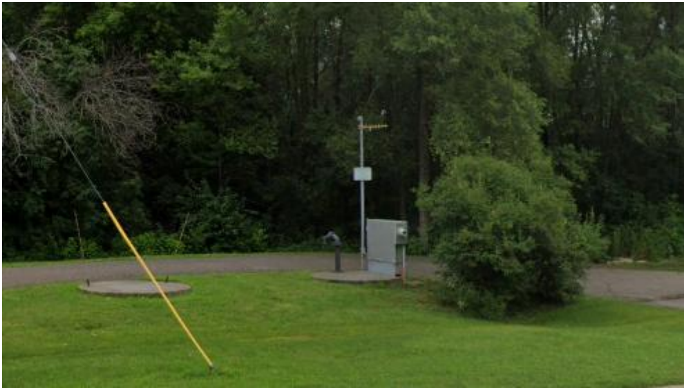
Figure 2.8: Brenner Sanitary Lift Station Site
