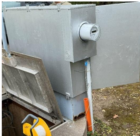
Control Panel/Utility Meter
