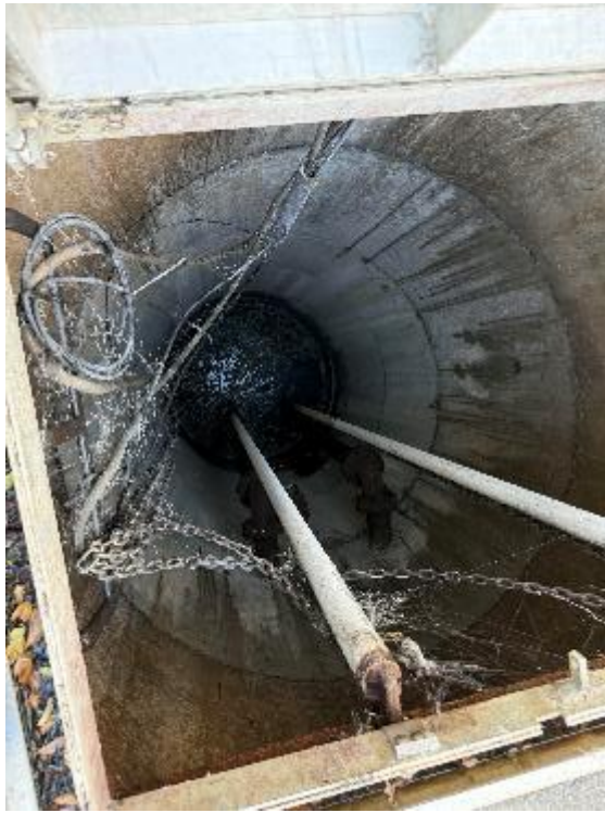
Figure 2.10: Brenner Sanitary Lift Station Wet Well
